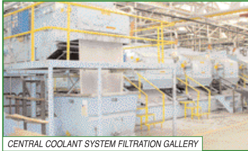
CENTRAL COOLANT SYSTEM FILTRATION GALLERY
